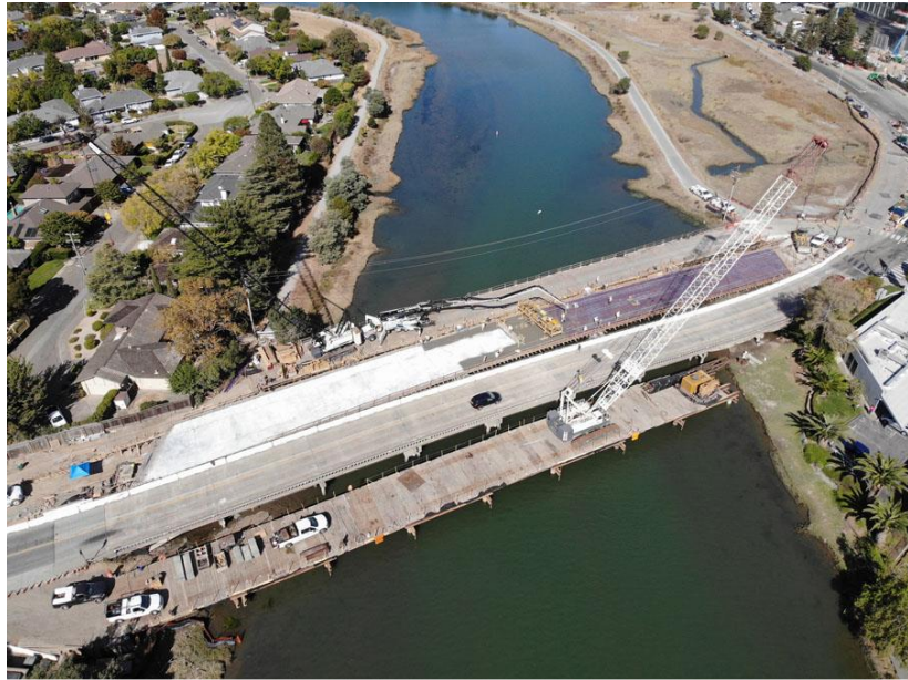
Replacing Bon Air bridge while keeping traffic flowing is a complex challenge. Photo courtesy of the City of Larkspur
