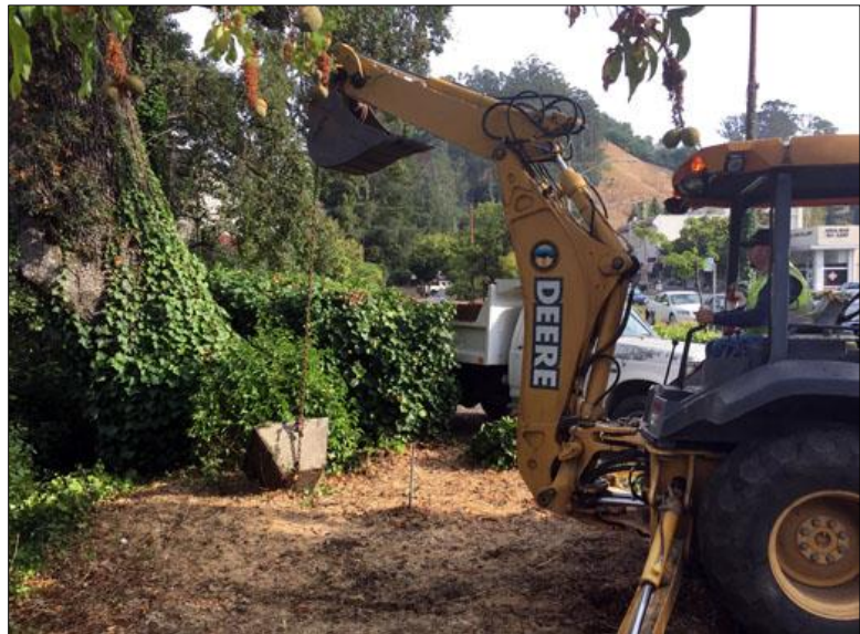
A concrete pier has just been lifted from the bed of San Anselmo Creek, for disposal. Photo by Gerhard Epke
