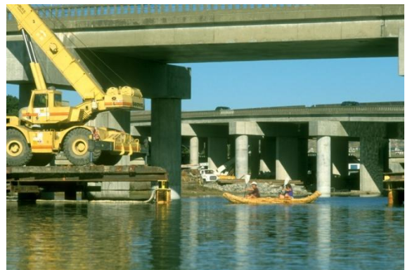
Unseen by travelers on Highway 101 overhead, life on Corte Madera Creek unfolds as a slower pace. Here a tule-reed boat has an encounter with a mechanized crane during work on the flyovers in 1997. Photo by Charles Kennard
