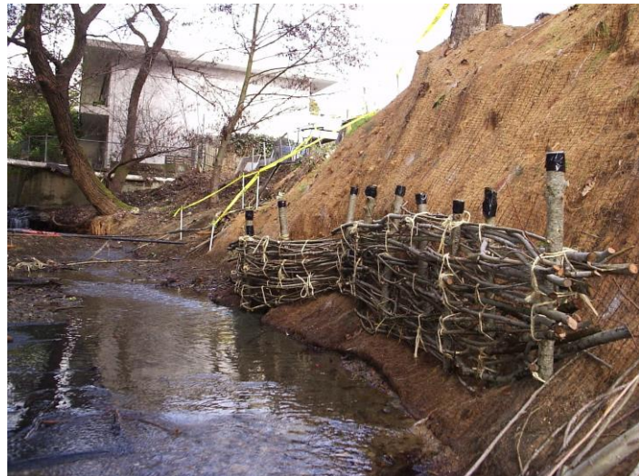
An erosion-control project on Fairfax Creek included a woven willow fence, whose posts will grow into bushes to protect the slope.
