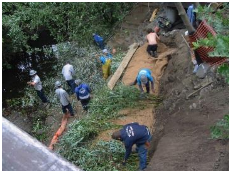
After the proposed removal of a concrete channel wall in Allen Park, an earthen creek slope will be contoured and planted in a similar way to what was done in Creek Park in San Anselmo several years ago. Photo by Harold Appleton
