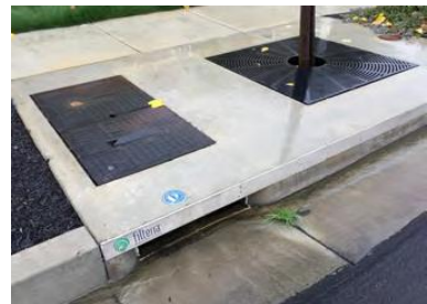
A Filterra storm drain inlet is located at the southeast corner of Rose Lane and Orchid Drive, in Larkspur. Photos by Sandy Goldman
