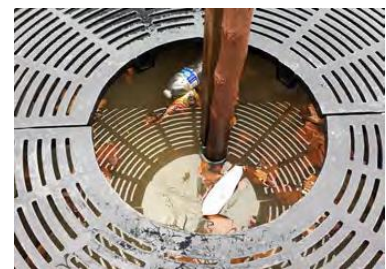
This close-up of the planted section of the Filterra unit shows accumulated trash, often discarded by students.
