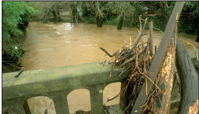
Neither high or dry enough: Nokomis Avenue bridge in San Anselmo was overtopped by the December 2005 flood, but with legal obstructions cleared, work will be able to proceed with watershed improvements to reduce flooding. Photo by Charles Kennard
