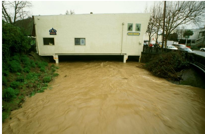
'Building Bridge 3' in San Anselmo seriously restricts high flows in San Anselmo Creek. The Town's water level gauge is located beneath the building. Photo by Charles Kennard
