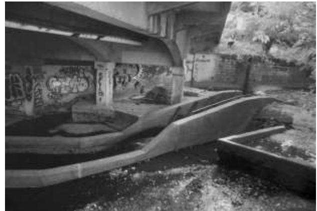
At the Saunders Avenue bridge over San Anselmo Creek, the present fish passage structure does not accommodate fish at all water levels, and a cross-creek sewer line contributes to local flooding. Photos by Charles Kennard
