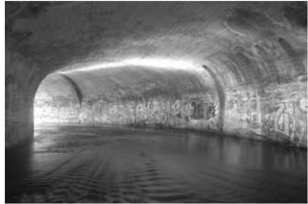
The almost flat floor of the long culvert under Center Boulevard at Lansdale Station prevents fish passage at low flows, while at high flows there are no resting places for migrating adults.
