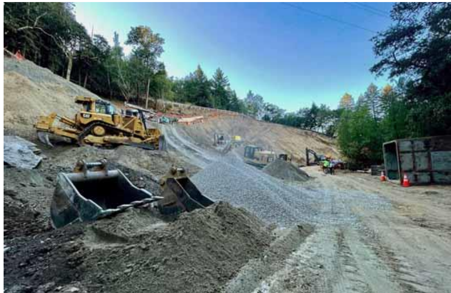
Major excavation is required to accommodate two new water tanks downhill from Sky Oaks Road. Photo by Gary Leo
