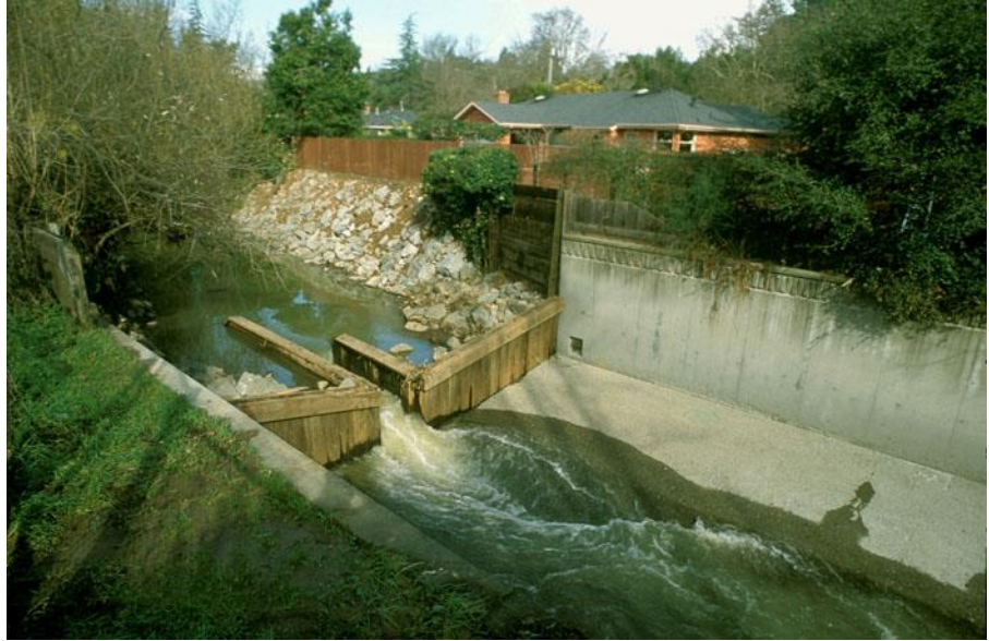
Where the concrete channel stopped, in 1971, behind the Ross post office. Photo by Charles Kennard
