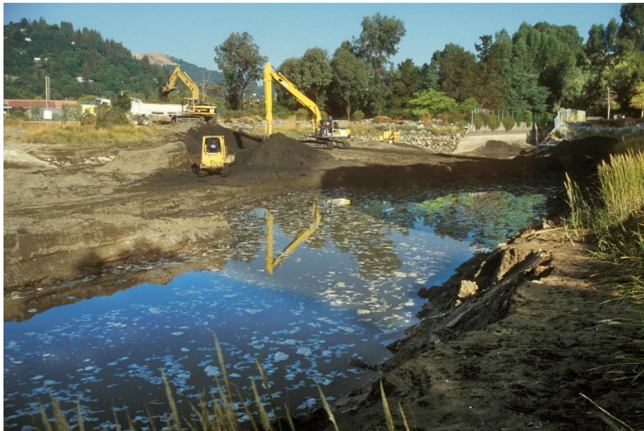
The 1998 dredging of Corte Madera Creek immediately downstream of the concrete channel required the building of two temporary dams. Photo by Charles Kennard
