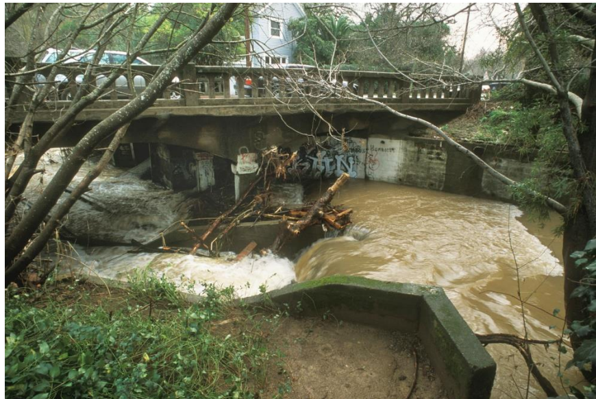
Existing concrete structures at the Saunders Avenue bridge cause multiple problems for people, property and migratory fish. Photo by Charles Kennard
