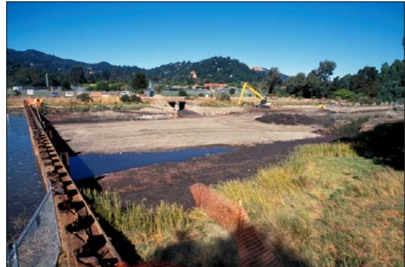
A temporary dam holds bay waters away from the mouth of the concrete channel
