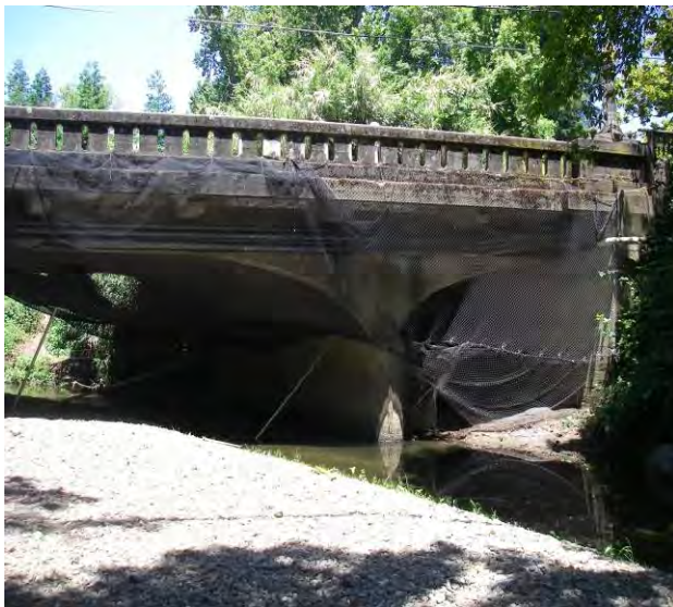
Figure A-6 picture SA_CM_37515_5 Corte Madera Creek at Lagunitas Bridge in Ross before construction. Ross photographs do not have 2006 versions.
